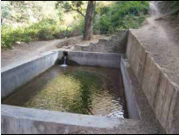
Fig. 15 (c) Water storage tank in a village
