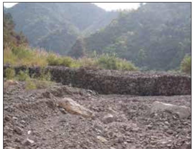
Fig. 15 (b) Infiltration gallery in village
