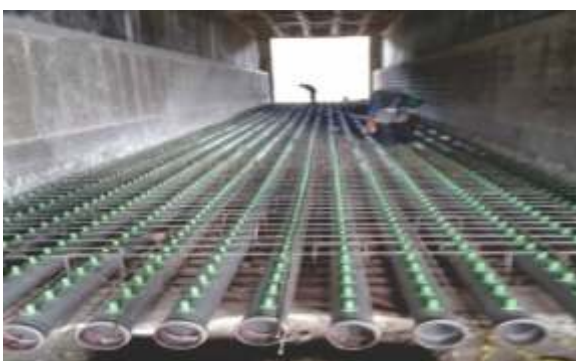
Fig. 48: Tunnel with iron grating (above) and with pipes & spigots (below) (under construction)
