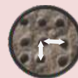
Fig. 49: Holes in Plenum
